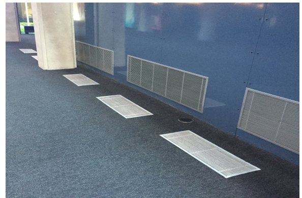
Figure 10: The only source of heat in the Davis Centre atrium.
